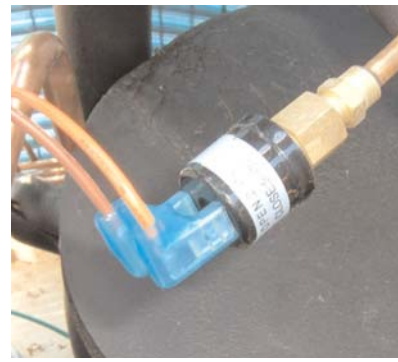
Low Pressure Switch (green) open 25 PSi closed 50 PSi
